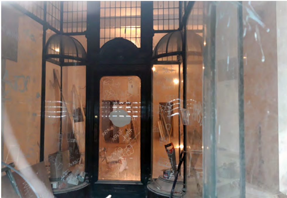
One of the two original shop fronts at No.103, preserved behind roller shutters
