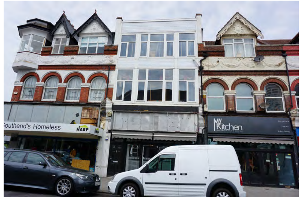
Poor quality rebuild of upper floors of No.157 Hamlet Court Road
