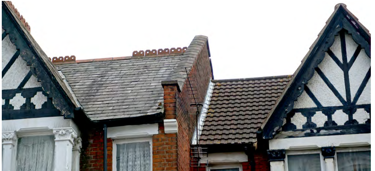
Original slates and some decorative ridge tiles on the house to the left, with unsympathetic concrete tile replacements on the right
