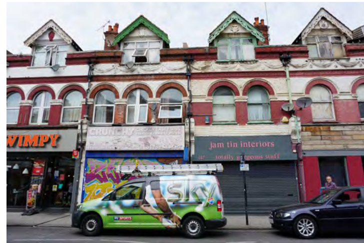
Nos.141-151 where the decorative condition is poor, architectural details have been lost and changes over time to individual units have eroded character and coherency
