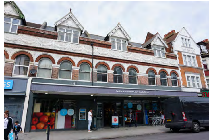
Nos.165-169 where the upper floors have been well-maintained, retaining original architectural details and materials, and creating a co-ordinated appearance
